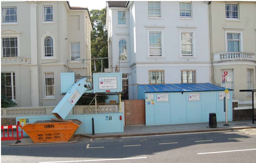
Figure 43. Example of restricted site access
