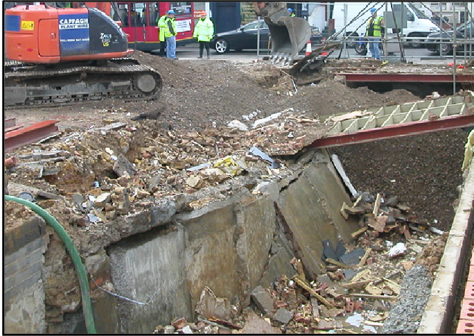
Figure 7. Wandsworth, South London during construction of a basement - effect of horizontal force from the ground on unrestrained basement wall
