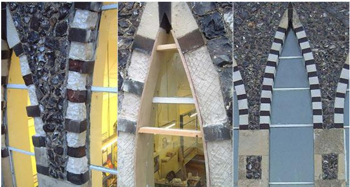
Left Damaged decorative stonework
