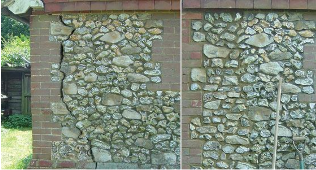
Left: Damaged masonry prior to repair
