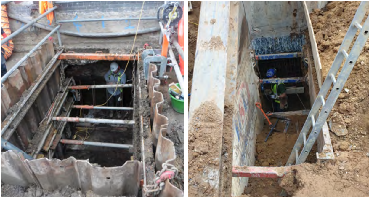
Photos 1 and 2 - Examples of good shoring to access pits for underpinning to external walls
